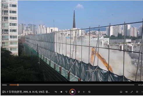
a) dust damage video data at construction
