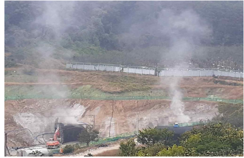
b) dust damage photo data at construction
